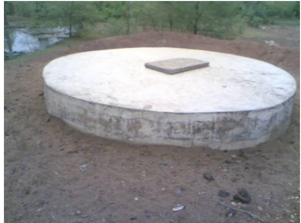
New water tank under the scheme
