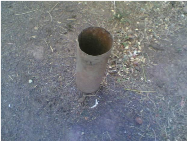
New tube well bore in the scheme
