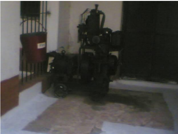
Generator repaired under scheme
