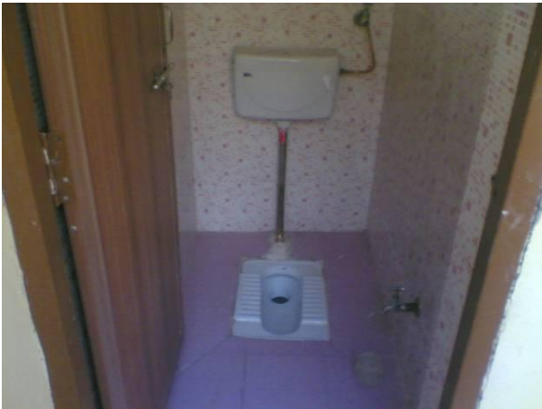
Toilets inside staff quarter
