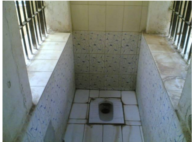
Night toilet inside the barrack
