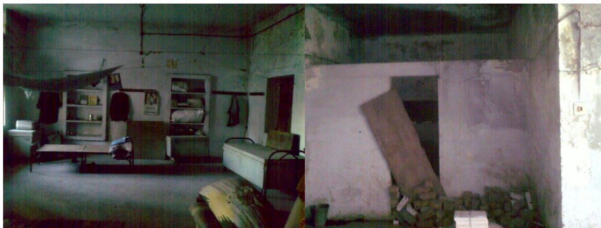
Figure 25: Condition of one of the better Police Barracks in Lucknow, UP
