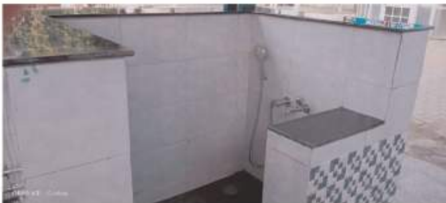
Bathing Cubicle with sanitary fittings
