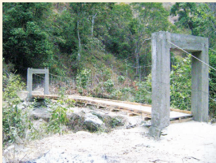
BADP – suspension bridge in between villages Nafra and Rurang In District West Kameng, Arunachal Pradesh
