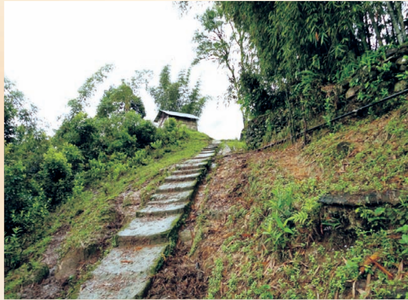
BADP – Construction of CC steps to Ngaming School, Tuting Block, District Upper Siang, Arunachal Pradesh
