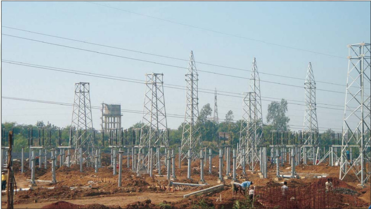
220/66 KV Sub-Station at Khadoli
