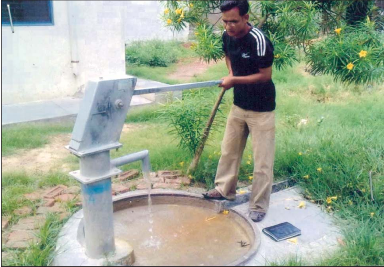
Installation of Hand pump under BADP in the High School Khatima, Uttarakhand
