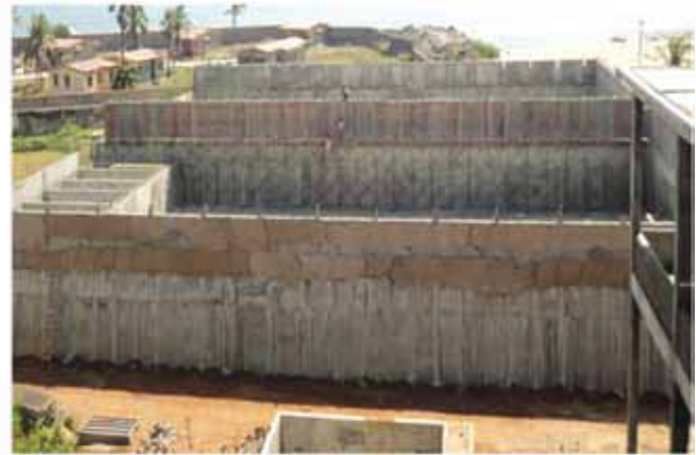
View of Sewage Treatment Plant-III @ Kanaganeri
