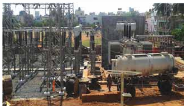
Venkata Nagar 110/11 KV Sub-Station
