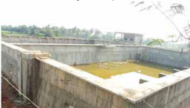
View of Sewage Treatment Plant-I @ Lawspet
