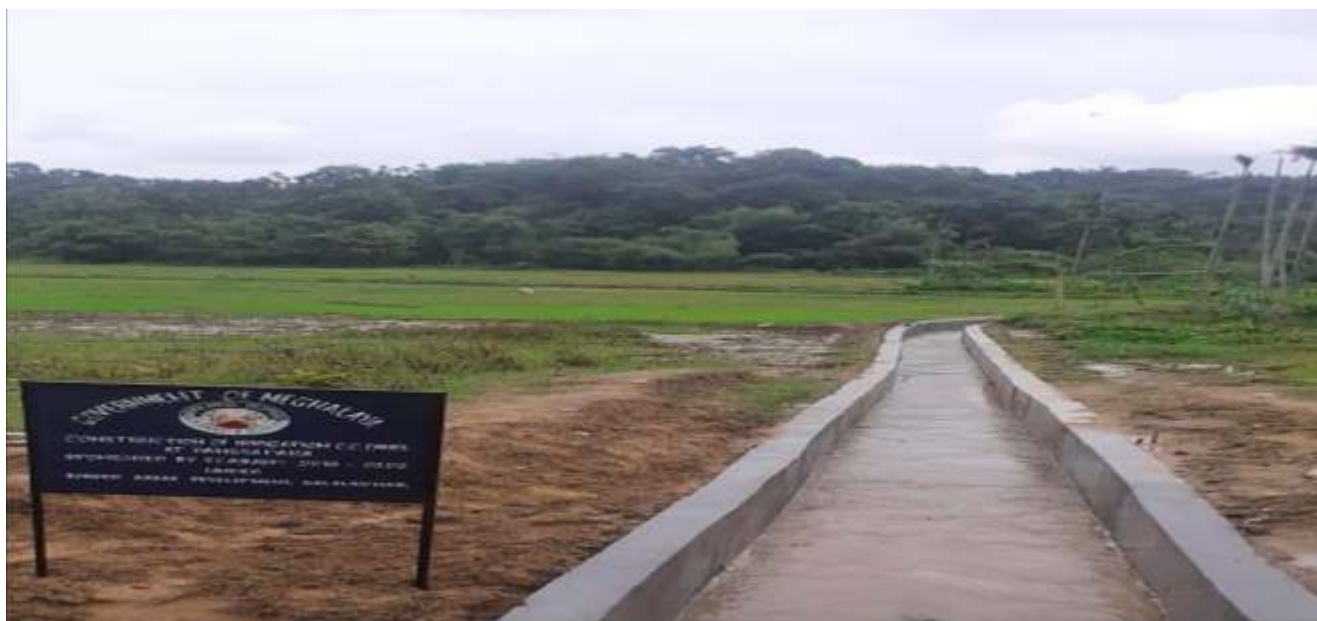
Construction of Irrigation Canal at Village: Dangsapara, Block: Kalaichar, District: South West Garo Hills (Meghalaya), Year of Completion: 2020-21
